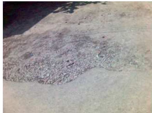
Figure 1: A deteriorated road surface.
